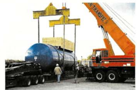
Coldbox ready to load on special low clearance trailer
